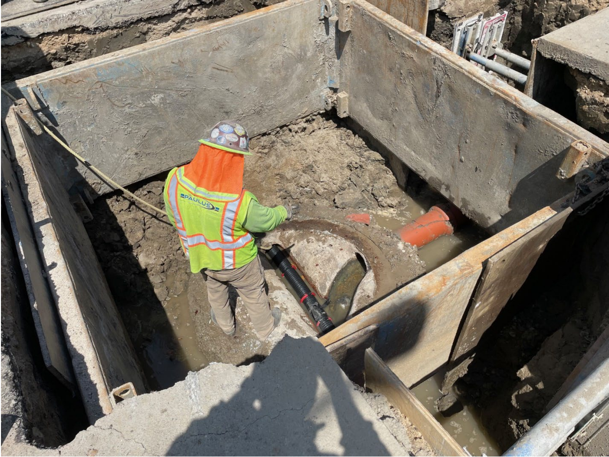
Photo #6 – 05/14/2024 – ground water issue after excavation
