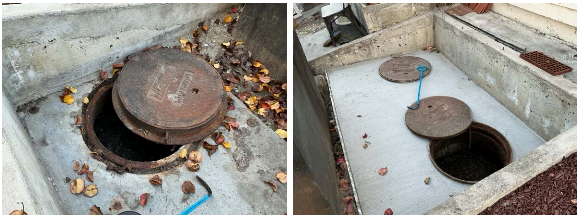
Com Tam Sa Bi Chuong: Lid unattached from the ground (before & after)
