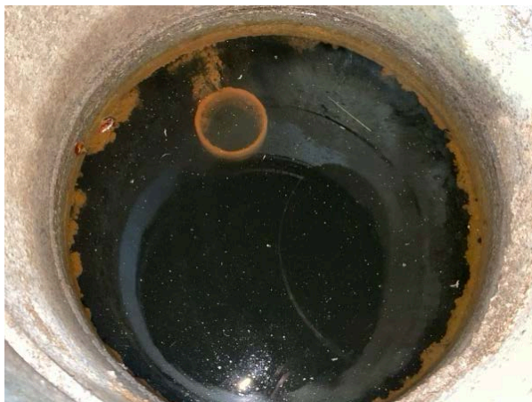
Quan 10 (interceptor disconnected)
