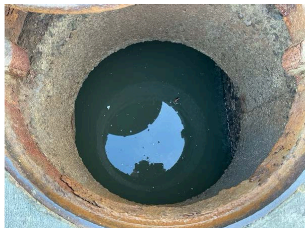
Red Sake & Sushi (interceptor disconnected)
